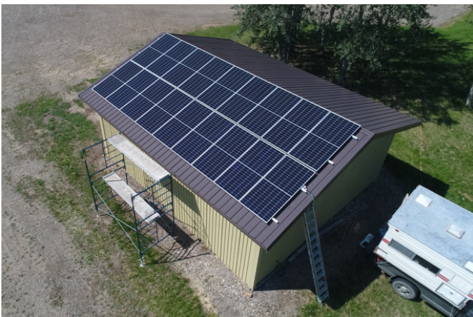
Stan Eason near Charlie Lake, BC now is the proud owner of a 7.9 kW grid-tied array mounted on his shop/garage.
