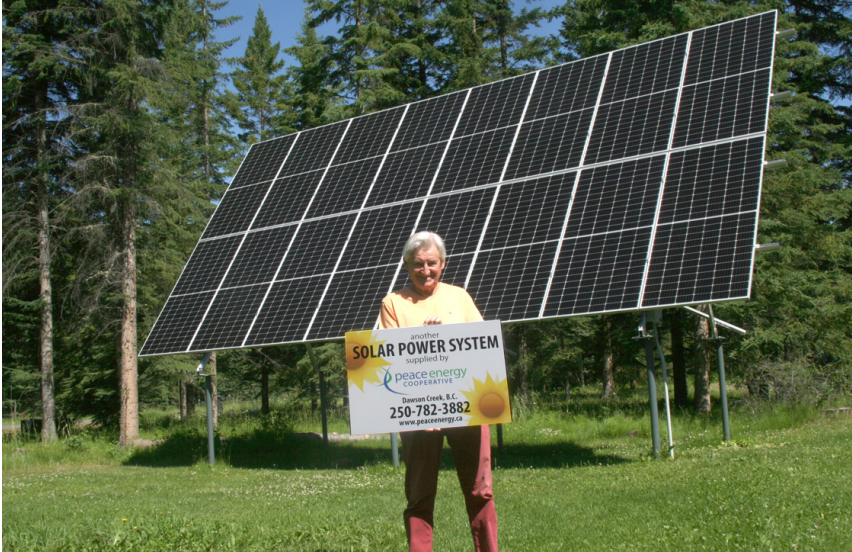
Christian Eschenburg stands in front of his new 7 kW grid-tied array on his rural property near Hudson's Hope, BC.
