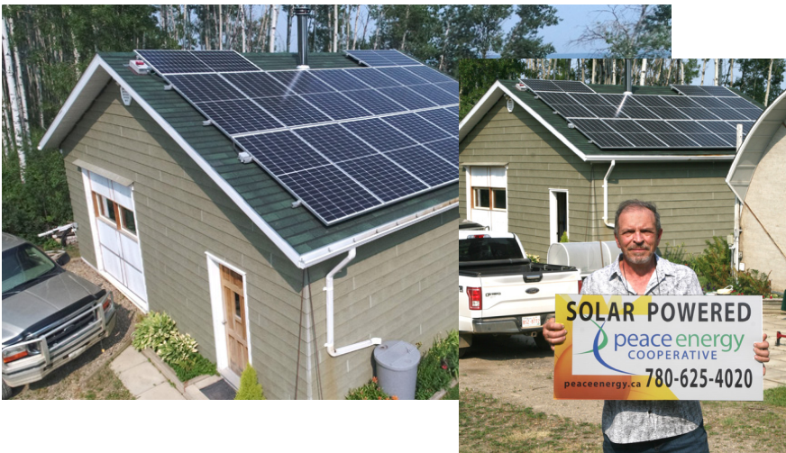
Left: We have just completed a shop-mounted 6.4 kW grid-tied array for Brian Hohner near Manning, Alberta. Going solar is another step in Brian's long-term effort to achieve a more sustainable lifestyle.
