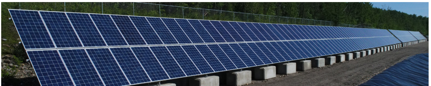
This solar array in Hudson's Hope, BC, provides about half of the power needed for their sewage treatment facility and should continue to do so with no moving parts and no pollution for at least 30 years.
