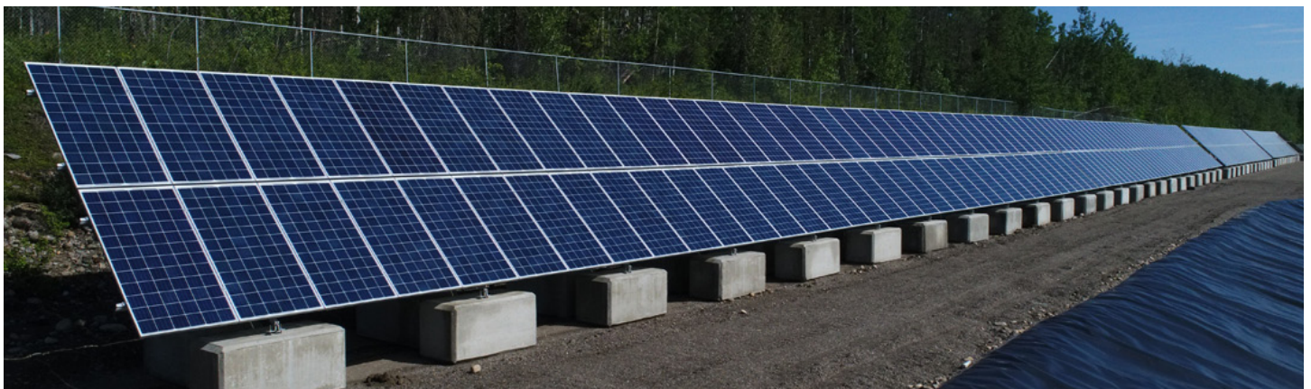
This 122 kW solar array provides about half of the electricity needed for the Hudson's Hope sewage treatment facilities. Solar array designed, supplied and installed by Peace Energy Co-op / Moch Electric Joint Venture, Dawson Creek.
