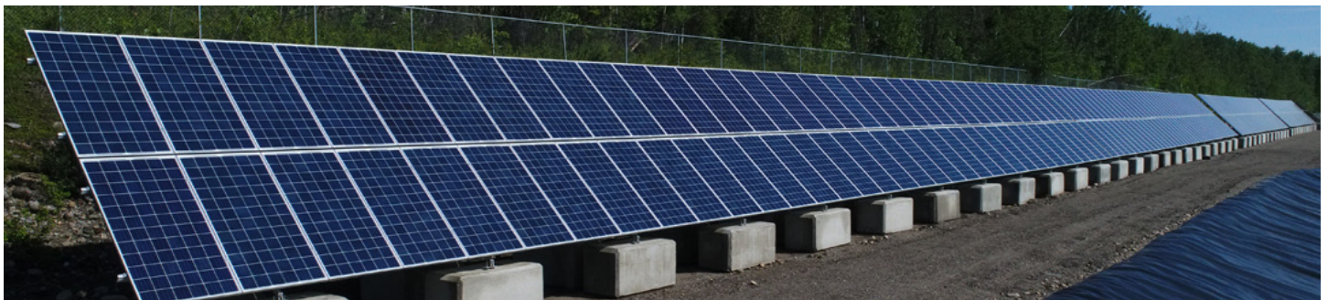
This solar array, another Peace Energy Cooperative project, powers the Hudson’s Hope sewage treatment facility with clean, low-cost solar electricity.
